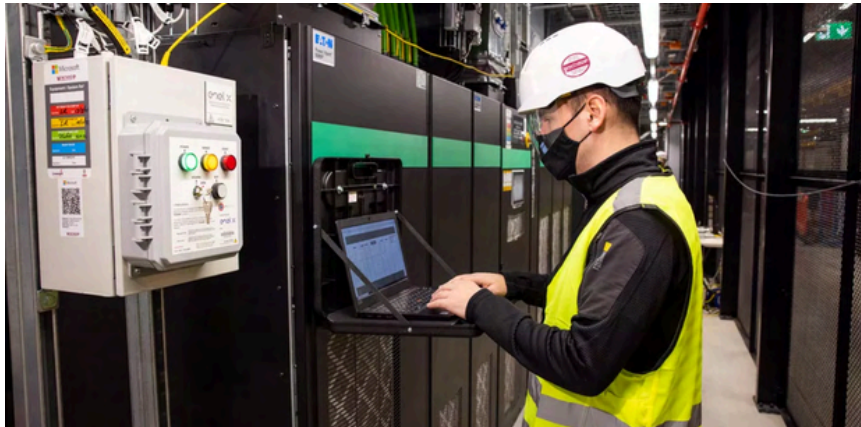
John Byrne, head of operations for Enel X UK & Ireland, performs a system test on the grid-interactive UPS inside a Microsoft datacenter in Dublin, Ireland. Photo by Naoise Culhane.
